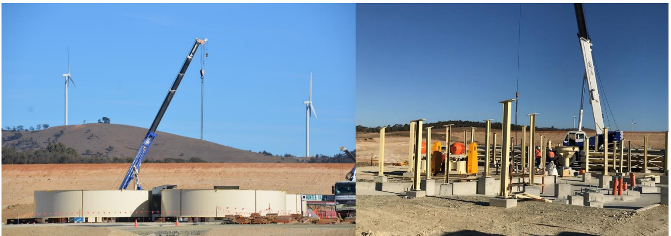
Figure 3: IsaMill feed tank strakes (left) and thickener tank support structure (right)
