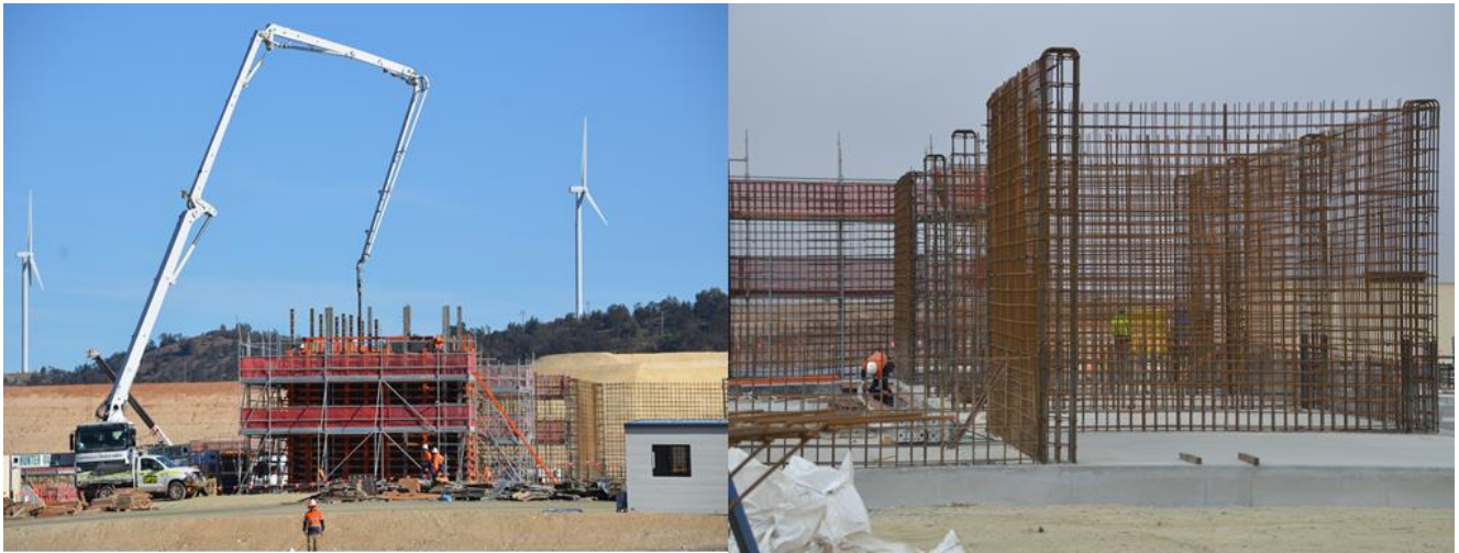
Figure 2: Concentrate handling area - reinforcing and concrete pour of the concentrate bay walls.
