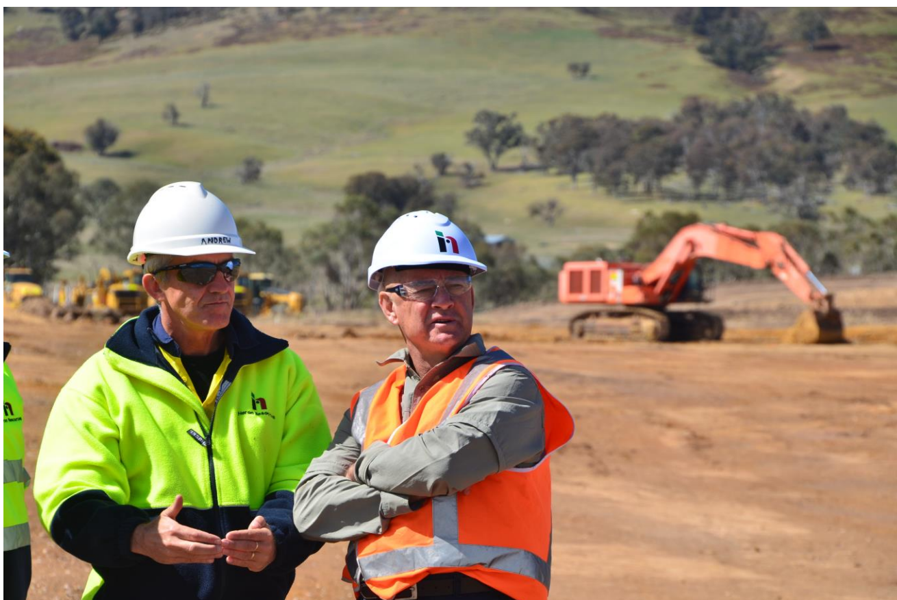
Figure 1: Heron's COO, Mr Andrew Lawry, and Chairman, Mr Stephen Dennis, discuss earthworks progress at the plant site.
